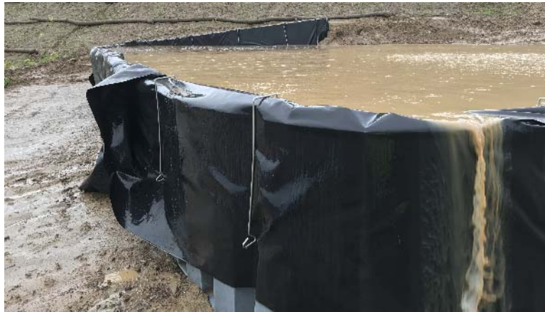
Figure 12: Basin MW-9 overtopping during a storm event.
