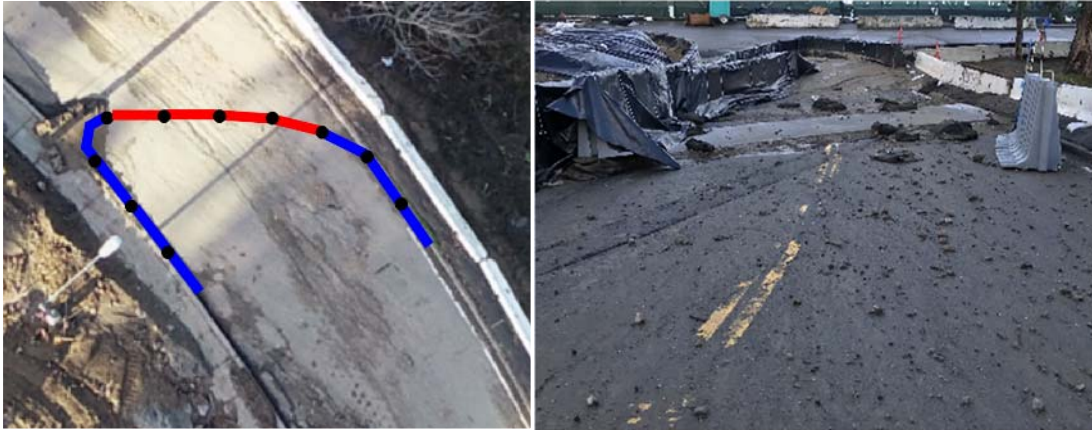
Figure 6. MW-3 initial configuration (left) and performance after first storm (right).
