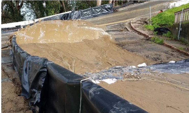
Figure 10. Basin MW-6 retaining 4 feet of sediment following a storm.
