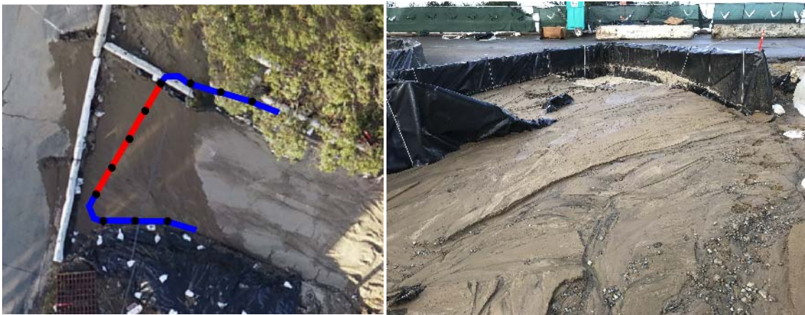
Figure 4. MW-2 initial configuration (left) and performance after first storm (right).
