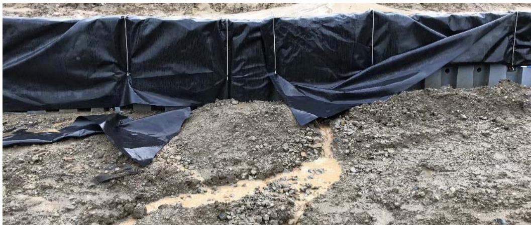
Figure 9. Seepage under the barrier wall.
