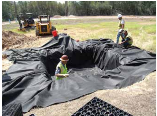
Figure 6: Roll out geotextile cut to fit the excavation in order to keep in-situ soils from migrating into the FocalPoint System. Geotextile strips must be cut generously in order to cover entire excavation on completion of the installation.
