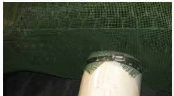
Figure 18: Cut "X" in Biaxial Mesh and Geotextile to accommodate outlet pipes and seal with stainless steel band clamps
